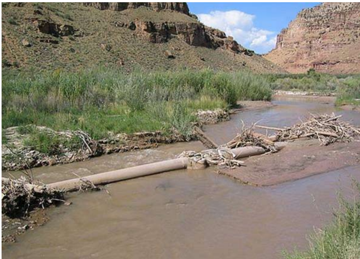
Figure 10. Lateral migration of this stream channel during high water excavated a section of pipeline under the floodplain that was several feet shallower than at the original stream crossing.
