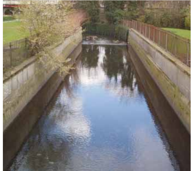
Cornmill Gardens: A river encased in concrete and disconnected from its surrounding environment 1
