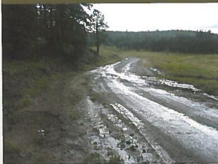
Figure 48. Inadequate surface drainage is a common problem across the area.
