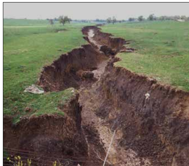
Figure 5. Poor riparian management has led to extreme downcutting in this creek. For reference, the block of soil closest to the camera is the size of a refrigerator. Photo by Kenneth Mayben, Natural Resources Conservation Service.
