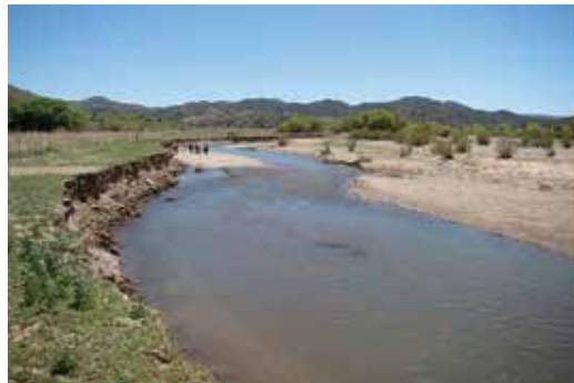
Figure 32. Evidence of bank erosion in an unstable channel could include slumps, sloughs, fractures, or slides. On this stream, the banks have eroded along long (several hundred meter), continuous spans. Eroded bank material is added to the channel and increases sediment load.
