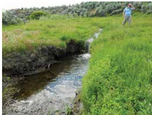
Figure 37. A headcut is moving upstream through a meadow, making the riparian area upstream of the headcut functional-at risk.
